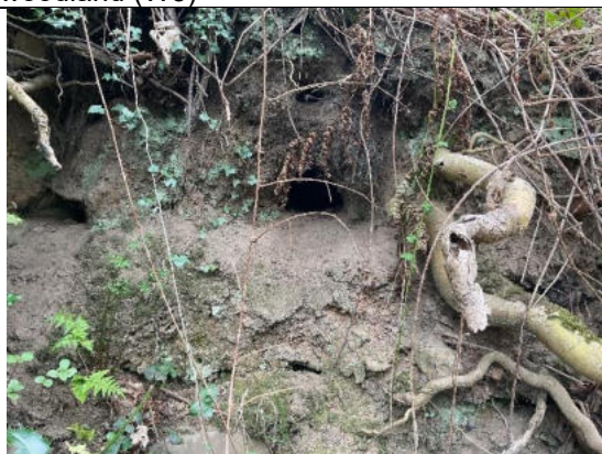
Photo 9: Exposed root system on Coltspool Burn.
