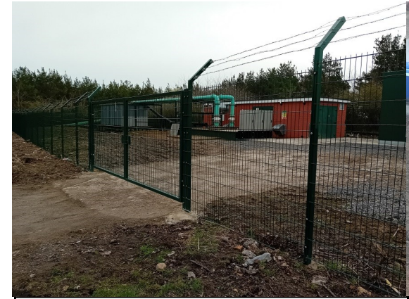
Photo 9— Mine Water Treatment Plant adjacent to site boundary in east of site.
