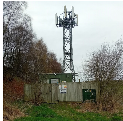
Photo 11— Telecoms adjacent to western area of site.
